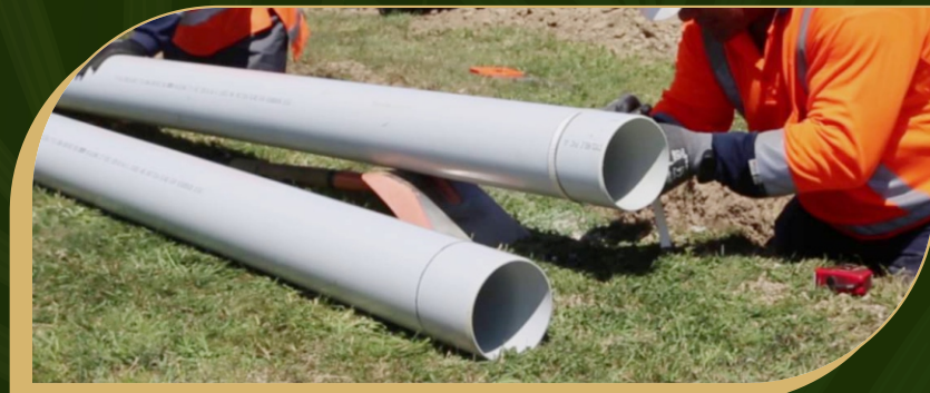
Water Pipe Line
