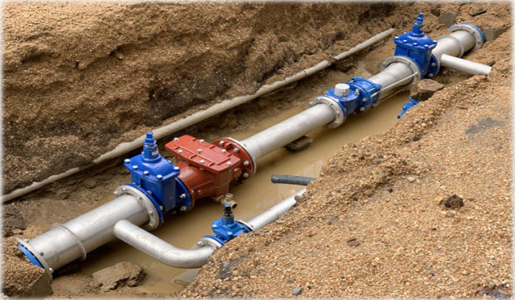
UNDERGROUND WATER-LINE EASY WAY OF WATER SUPPLY.
