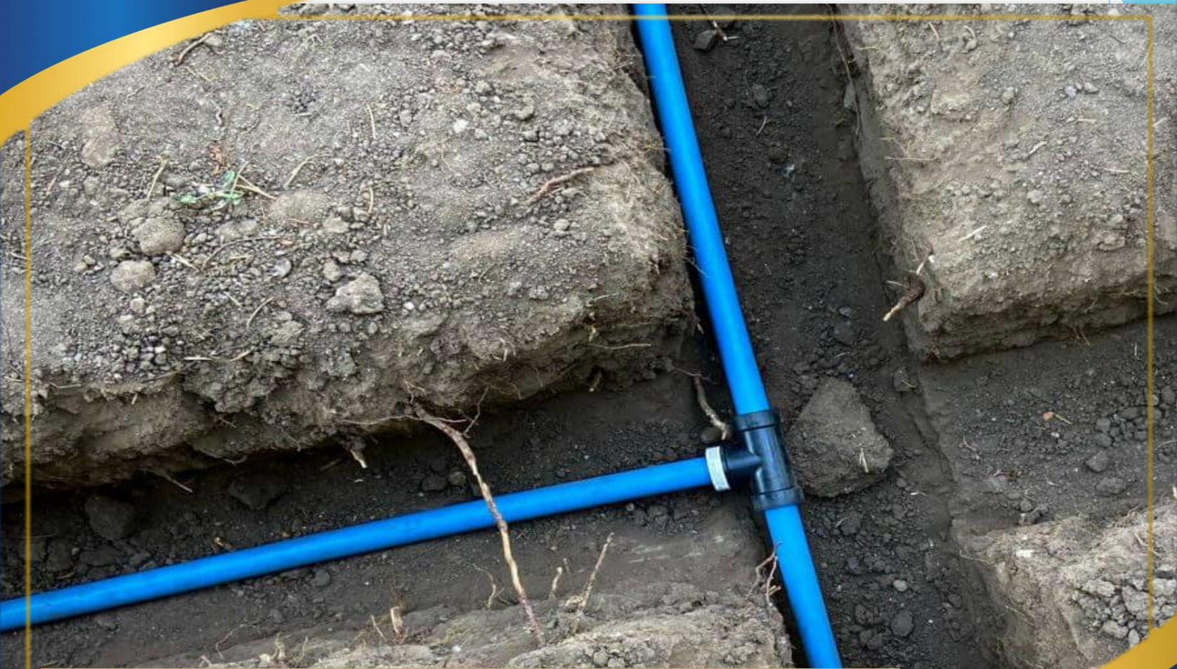
Underground Water Supply Pipe Line
